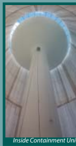
Inside Containment Unit
