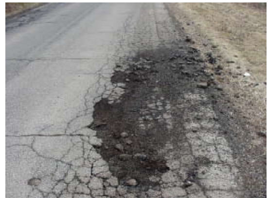
Section of deteriorated pavement
