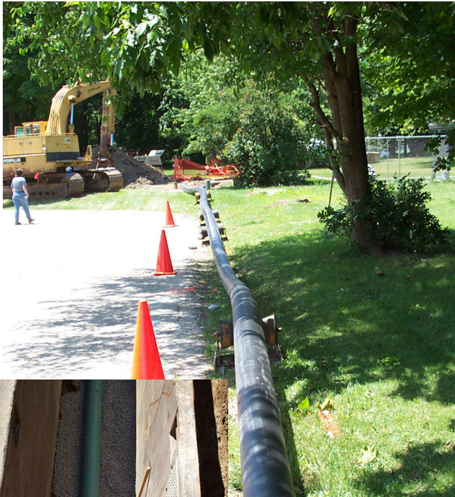
8" diameter gravity sewer
