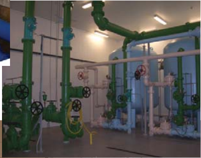
Cation Exchange Units
