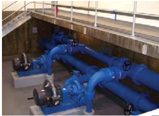
High Service Pumps
