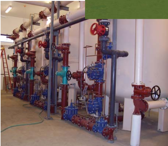
Three 8-Foot Diameter Cation Exchange Units
